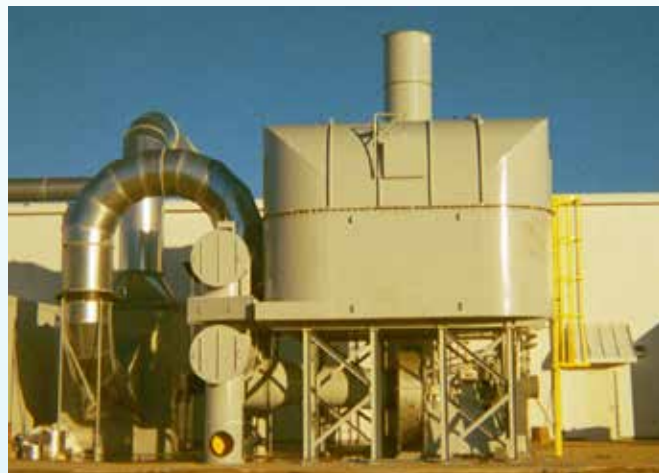
Auto Paint · 45,000 scfm · 2 Chamber unit
