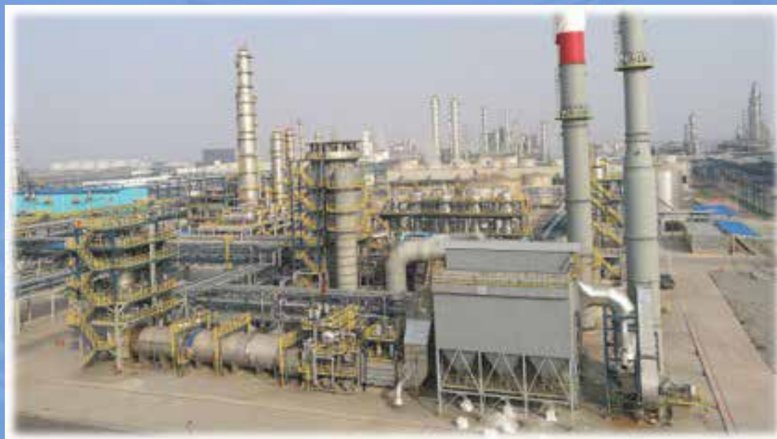
PCC successfully executes large, complex air pollution control trains.
